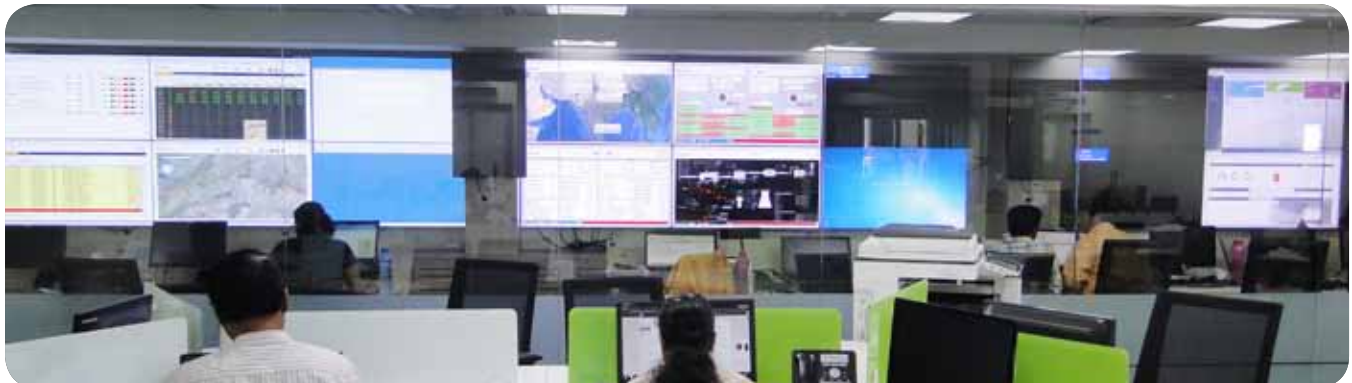
SCADA Room for Plant Operations Management
