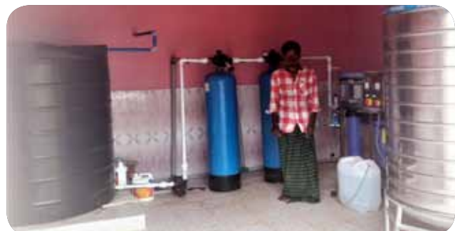
RO Plant at Cholasamudram
